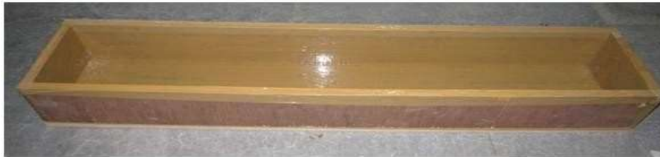
Figure 2: Completed formwork with sharp edge
