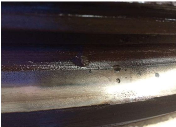
(c) Denting and corrosion
